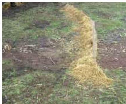
A fairly typical silt trap made from rice straw and old wire not long after installation.
